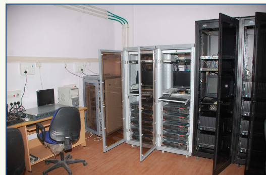
Computer Server Room
